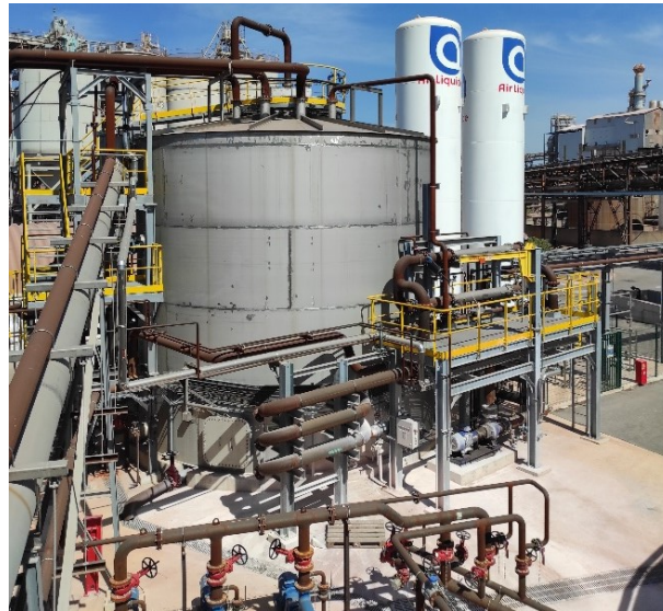
Figure 7. CO 2 neutralisation unit.
